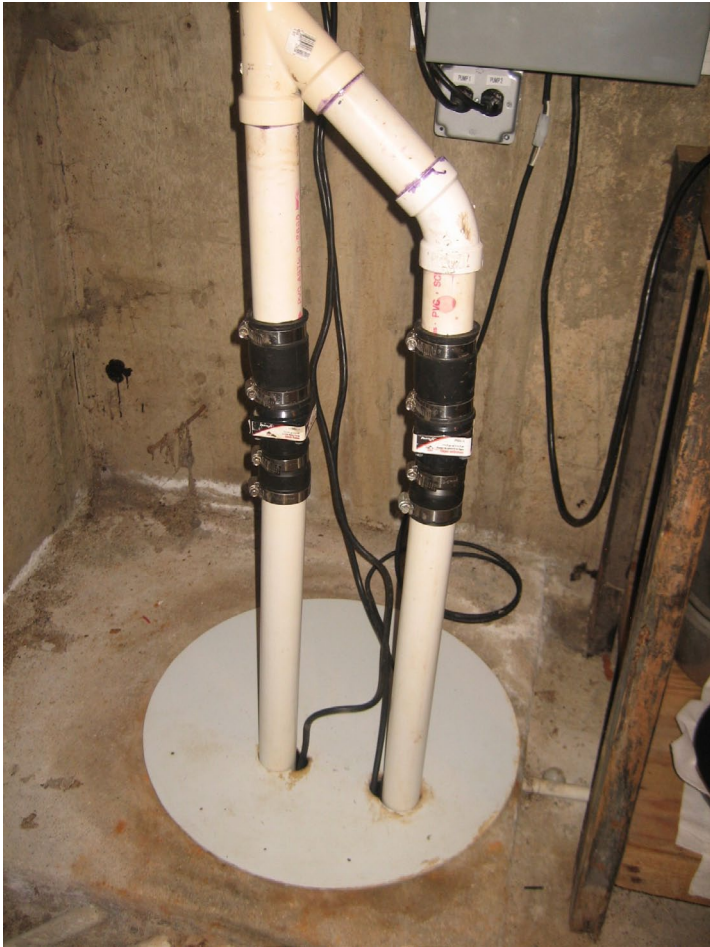
Figure 7 — Two identical ½ HP pumps — each with its own check valve reside in the sump. These are consumer-grade pumps that can be easily replaced upon a failure. A high-level float switch was added to detect a failure of a pump to run.
