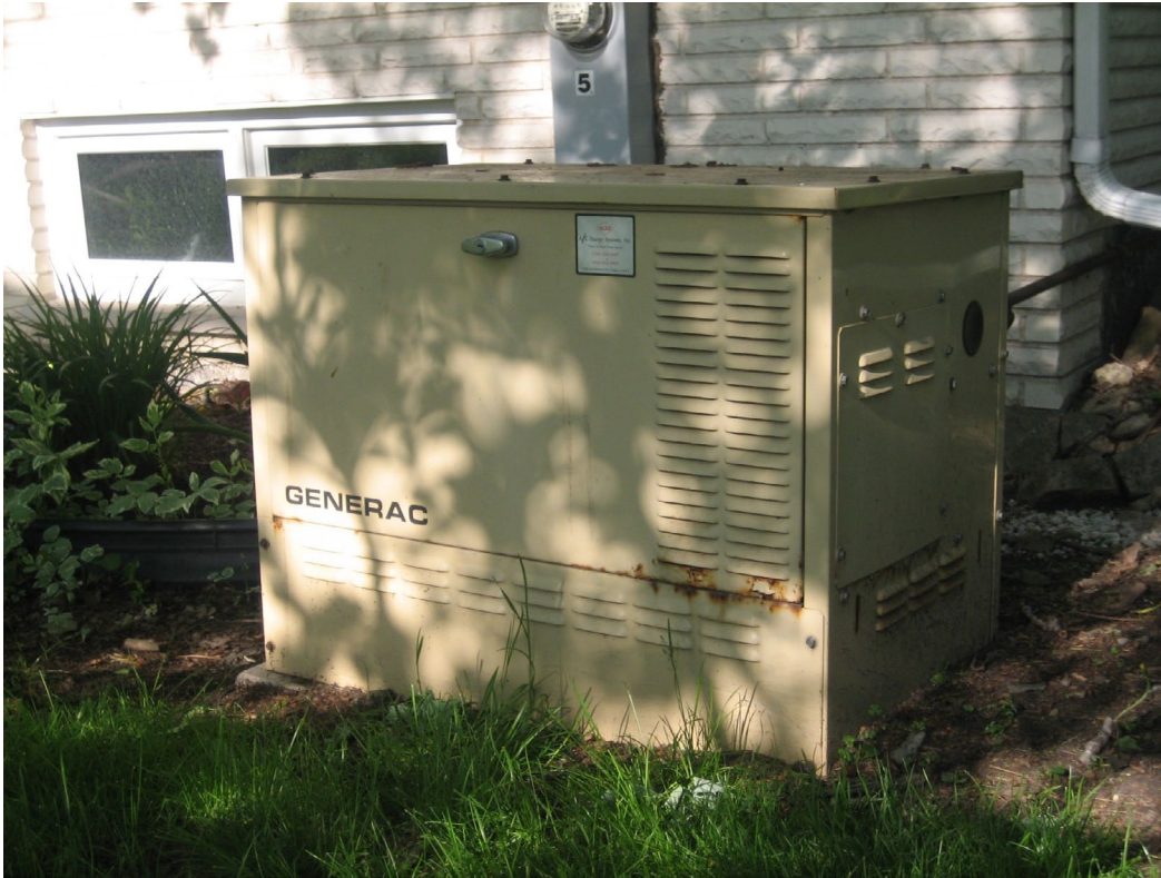
Figure 5 — A Generac 8 kVA natural gas-fired standby generator is the only source for backup power. Its weekly exercising is monitored by the BASremote.
