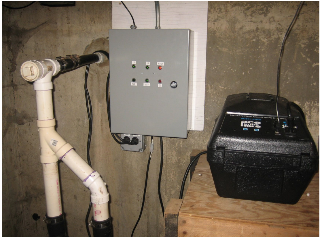
Figure 8 — Wall-mounted sump pump panel with battery case nearby. Pumps plug into a duplex receptacle alternately switched by interposing relays. An Ethernet connection is made to the homeowner's residential gateway.
