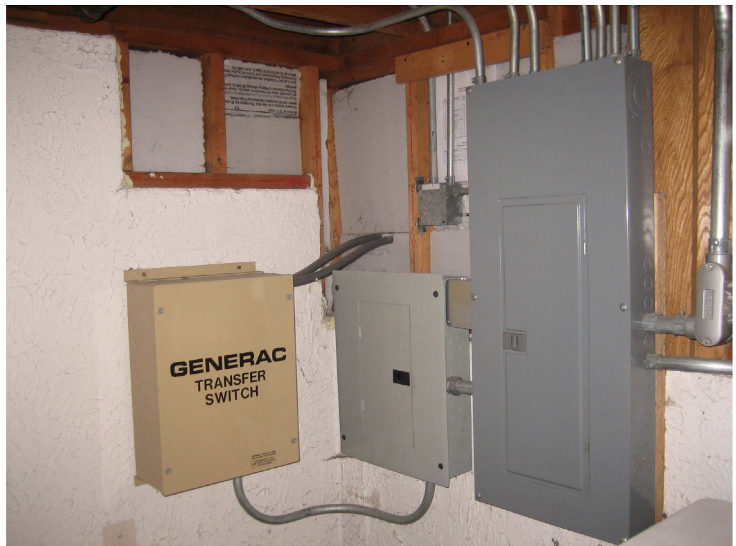
Figure 6 — An automatic transfer switch feeds the smaller distribution panel when there is a loss of utility power. Only critical circuits are backed up which includes the sump pump.
